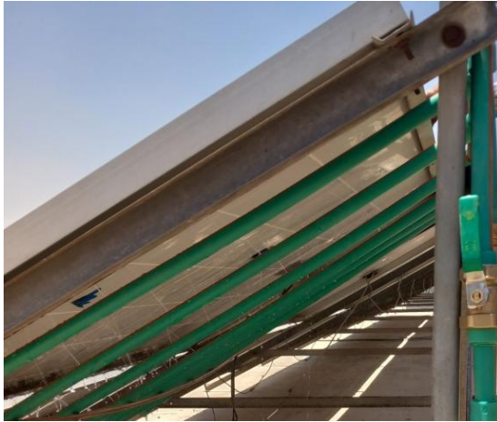
Fig. 1: Water back cooling system for PV panel
